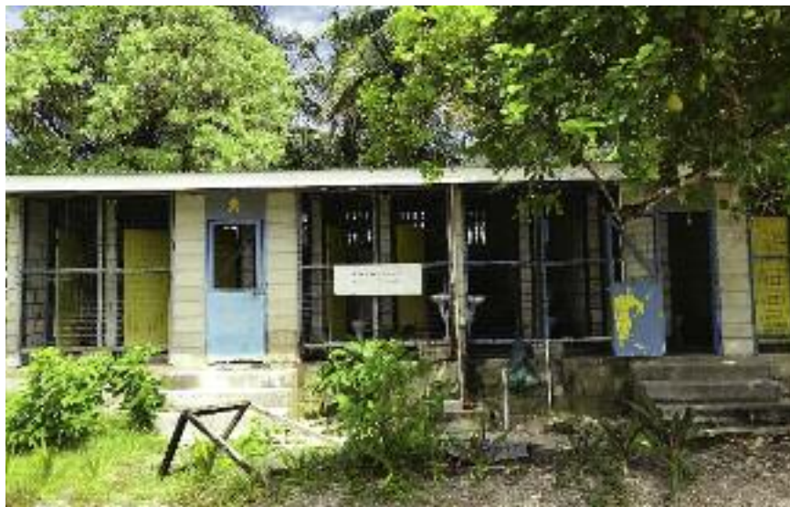
The senior girls' toilet block in need of urgent repair
