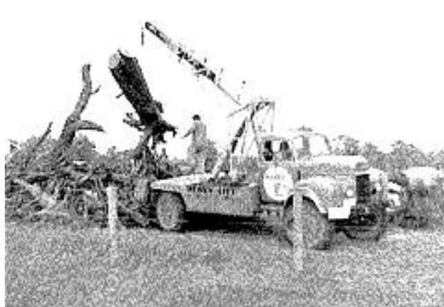
1961: Work begins on July 15 to clear ground for college oval. Kevin Sauer in charge of proceedings
