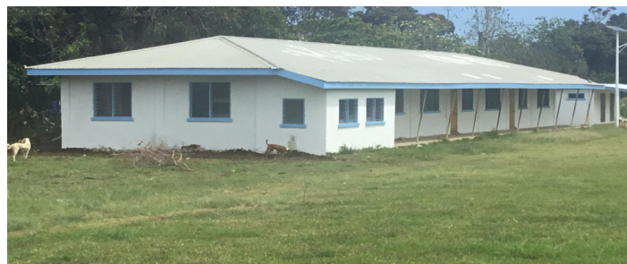
Newly restored building at Sts Joachim and Anne Kindergarten, ready to receive students.
