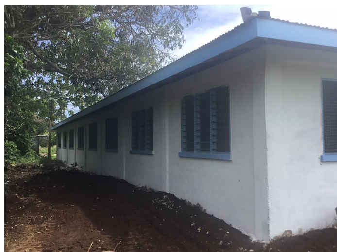
Back view of Sts Joachim and Anne Kindergarten after the much needed renovations.
